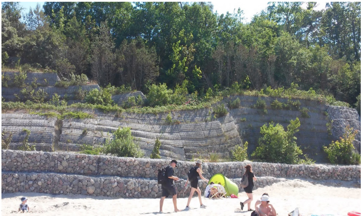
Fig. 3. Effect of groundwater on cliff bank reinforcement in Jastrzębia Góra - observation during field exercises in June 2022.
