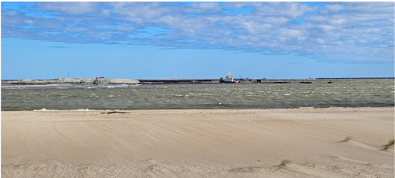
Fig. 1. Expansion of further quays of the Northern Port in Gdańsk on Stogi Island – by backfilling the surface of the sea area – May 2023.
