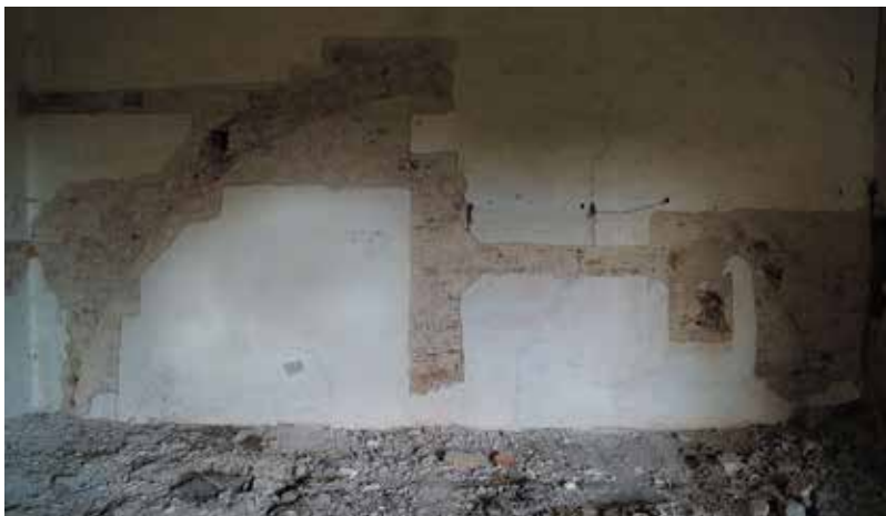
Fig. 7. Removal of plaster from the east wall on the second storey of the castle at Swobnica revealing the outline of the pier that once supported the ribbed vault of the former chapel (photo: K. Wroński)
