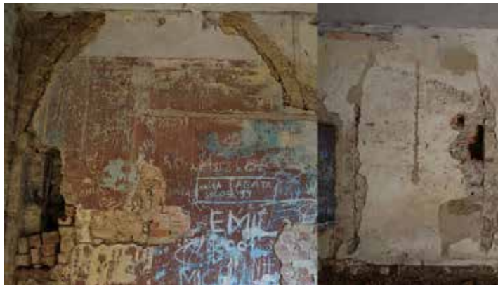
Fig. 5. Bricked-up windows of the former chapel at Swobnica. On the left is the west window seen in the outer elevation, and on the right – the east window seen in the interior elevation (photo: K. Wroński)
